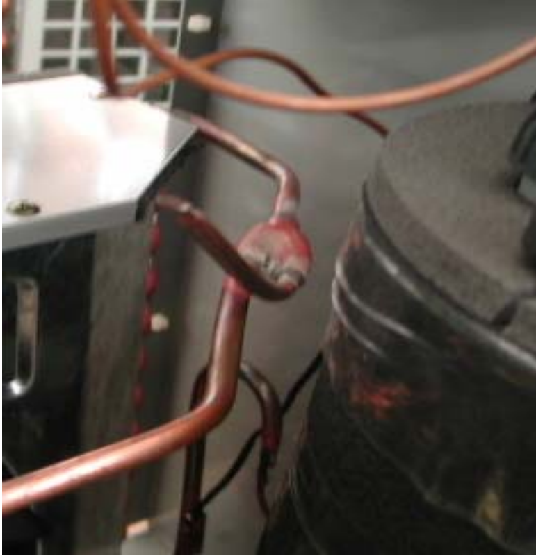
Pict.8: Y joint for service pipe and there isn't any dry filter.
